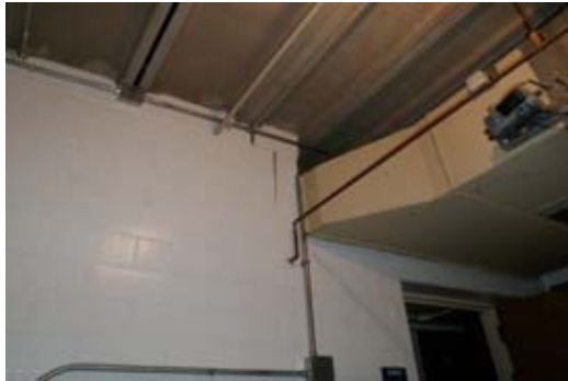
Figure 7, cracked CMU in 1952 bldg mech penthouse.
